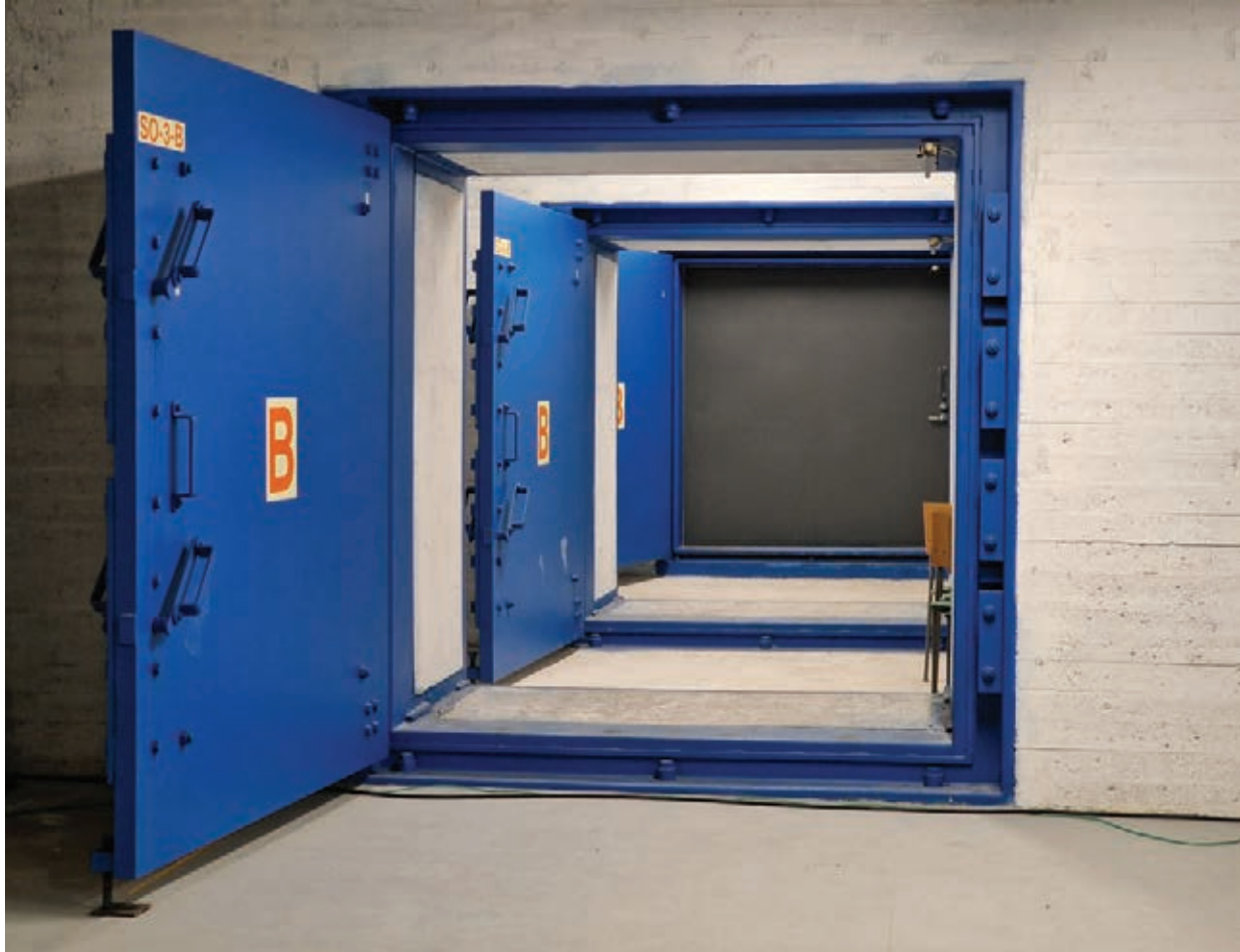
Helsinki underground civil defence shelters
