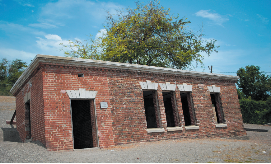
FIGURE 6.3 The Giddy House in Port Royal, Jamaica COURTESY OF THE JAMAICA NATIONAL HERITAGE TRUST
