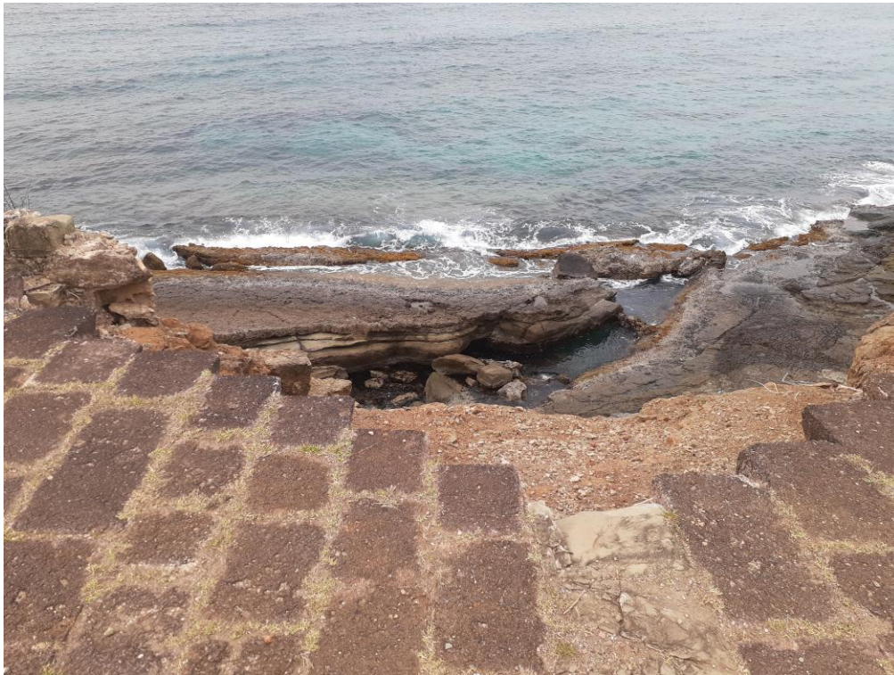
Figure 11. Missing Wall and Eroding Components at Fort Berkeley
