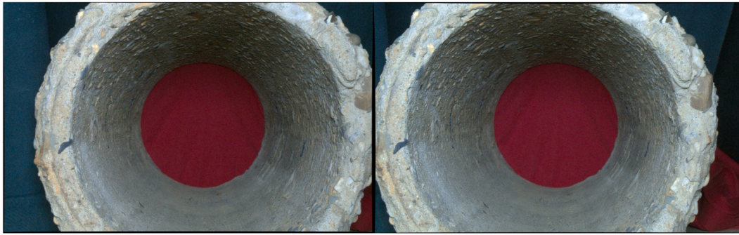
(a) A typical naturally aged cylindrical sewer pipe.
