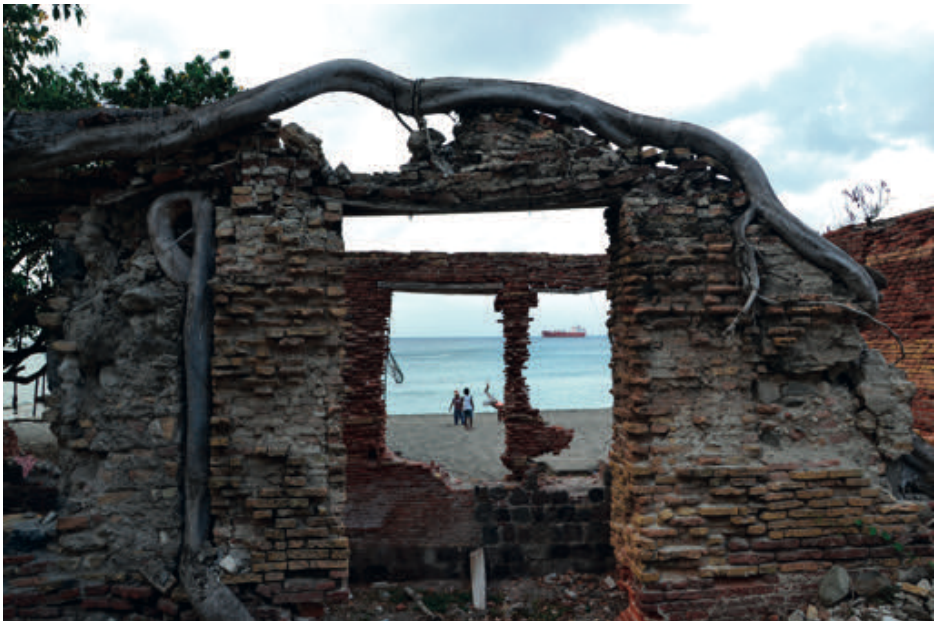
Figure 2. Colonial ruin on St. Eustatius in Lower Town, being engulfed by trees.
