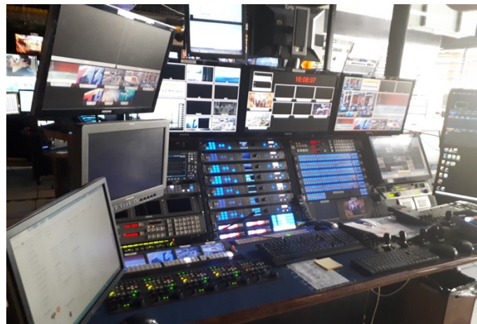
Figure 1. Production control room at Canal 13. Photo: Tomás Dodds during fieldwork.
