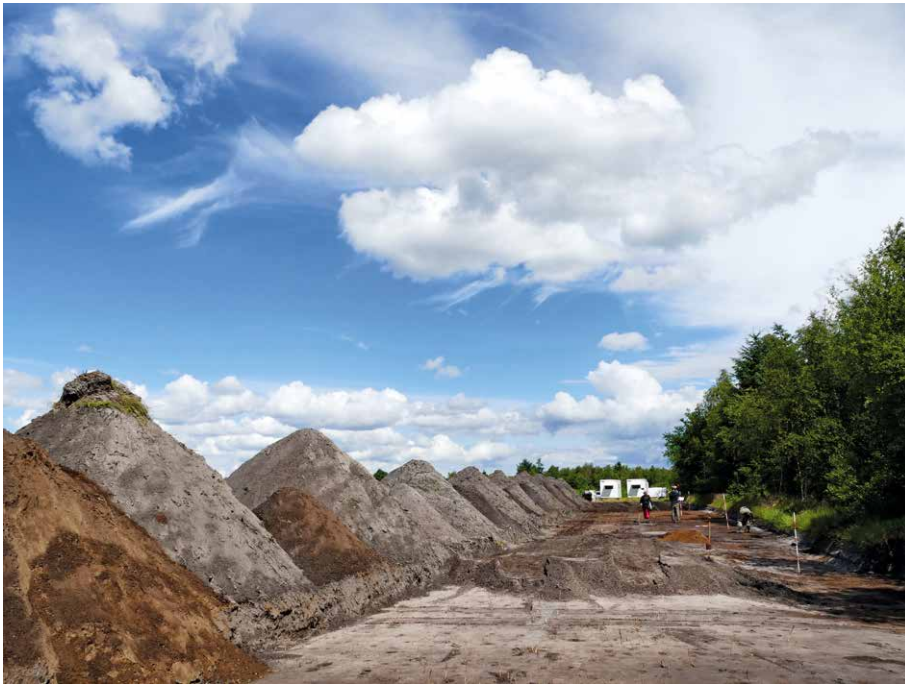
Figure 10.1. Excavation of the palisade at Boest in June 2016, carried out by Museum Midtjylland with assistance of the Economies of Destruction team. Photo: Marieke Visser.
