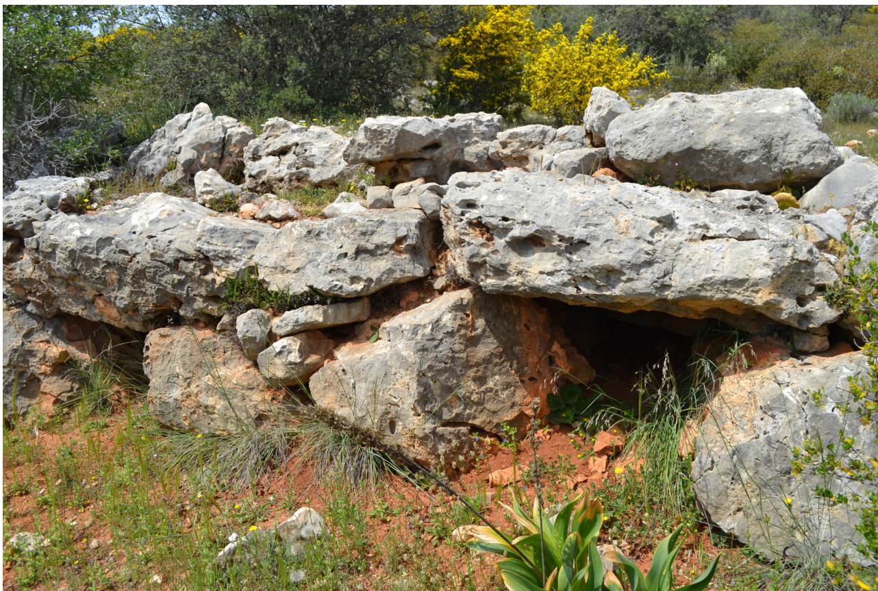
Figure 4b. Detail of Mycenaean highway M1: two of the dozens of culverts along M1 facing the terraces or valley downslope in 2018 (figure A. Brysbaert).
