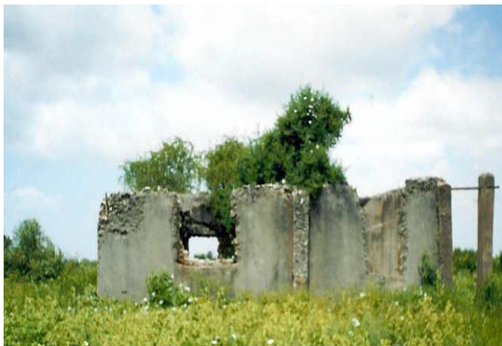
Photo 8.1 A burnt house at Tarasaa village
