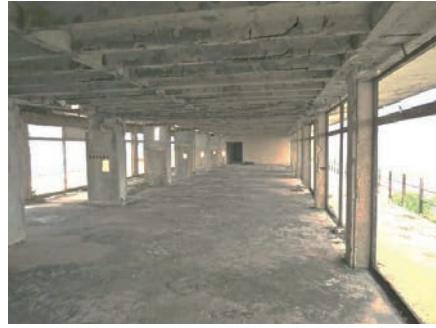
Illustration 28b All that remains of the Ducor Hotel is a concrete shell
