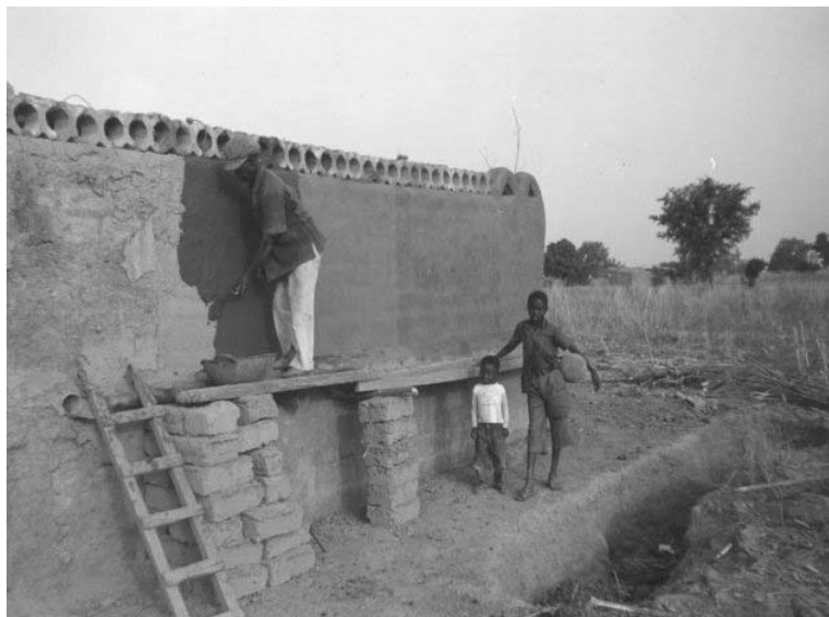
Photo 1 Mr. Kontana plastering the wall of his compound with sand and cow dung
