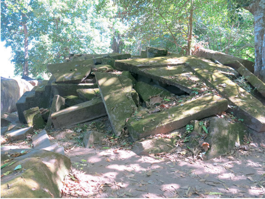
Figure 8: Collapsed stone cella, Vat Phu Temple Complex (author photo).
