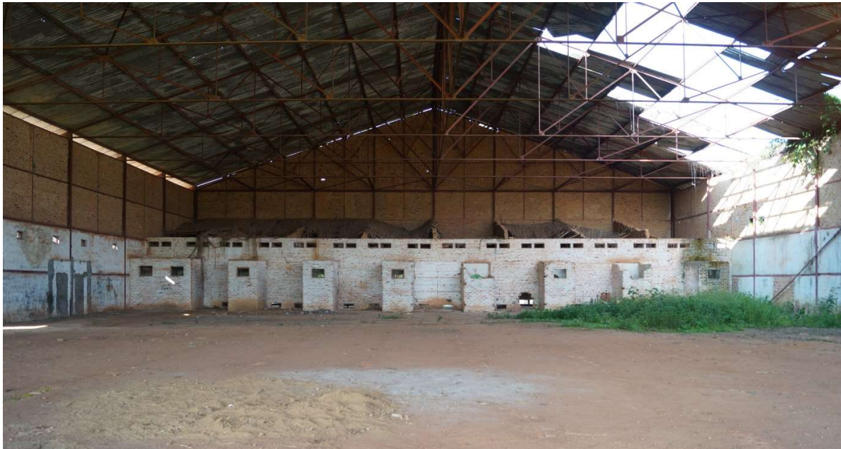
Figure 43 Bombed hangar at Libenge Airport Notice the hole at the top right (Photograph by Mirjam de Bruijn, Libenge, 11 June 2014)
