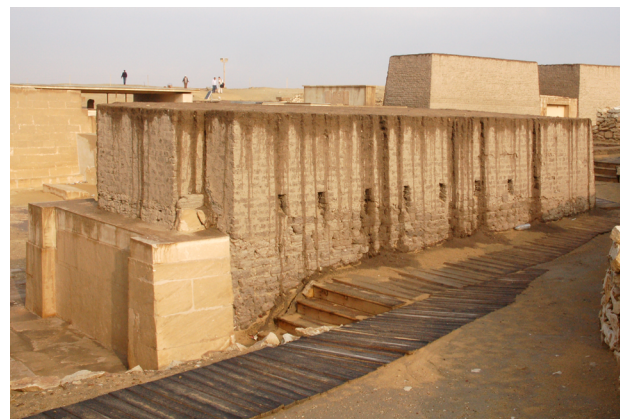
Fig. 36: Effects of the severe rainstorm of April 24/25 on the north section of the easternmost pylon of Horemheb’s tomb. Photo by Nicholas Warner/Leiden-Turin Expedition to Saqqara.
