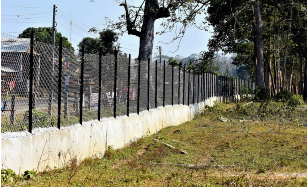
Figure 5.7 An example of the mesh wire fence communities prefer to construct along the forest-settlement border. The fence has a concrete base of about 2 feet and 5 feet tall mesh wire anchored to the iron poles set in a concrete base.
