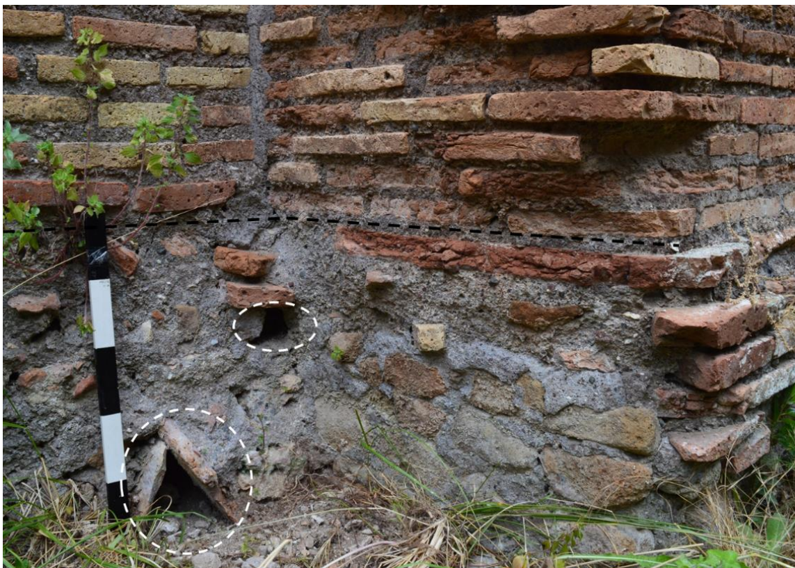
Figure 4.127: View looking west at the eastern side of room 8 of building IV, ii, 4. The cappucina drain 89 and the southern end of channel 116 are indicated by the dashed circles. The black dashed line indicates the transition between the foundation and the upper courses of the wall.
