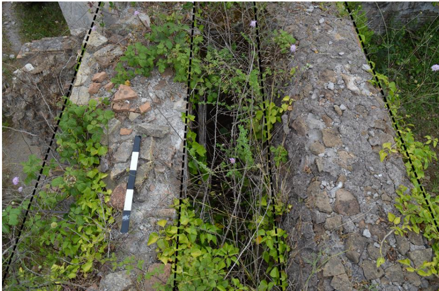
Figure 4.135: View looking south at doubling of walls between the cistern (right side) and the Terme del Faro (left side). The gap lies between these two walls.
