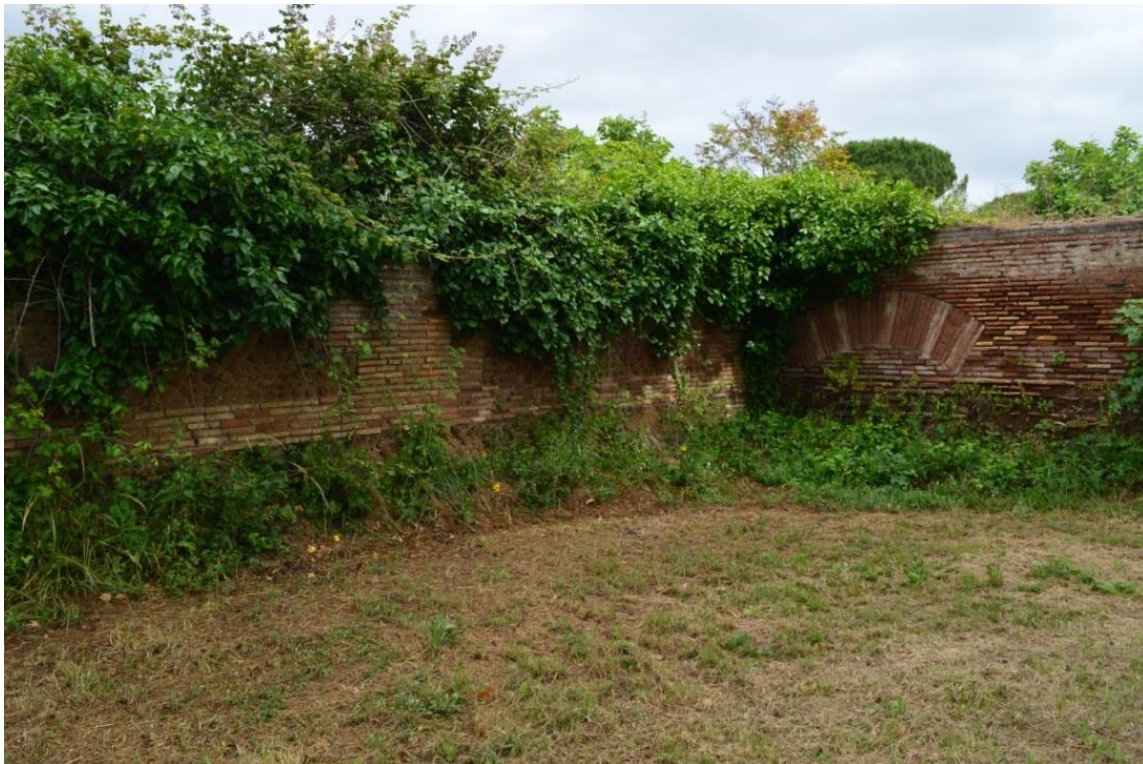
Figure 4.156: View of the external east face of building IV, ii, 8 where it intersects with the south wall of building IV, ii, 9.
