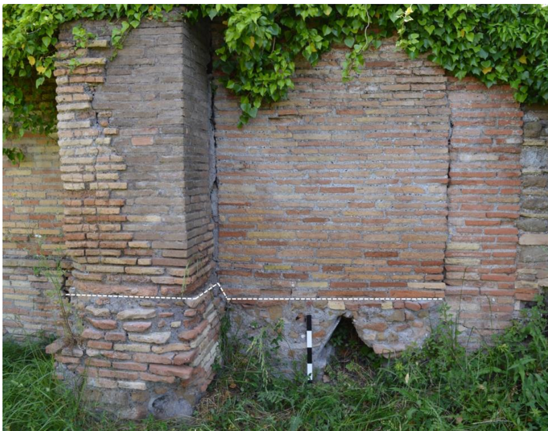
Figure 4.170: View looking east at the cappucina drain (feature 63) going through the west wall of room 1 in IV, ii, 12. The dotted line indicates the line between the foundation and superstructure.
