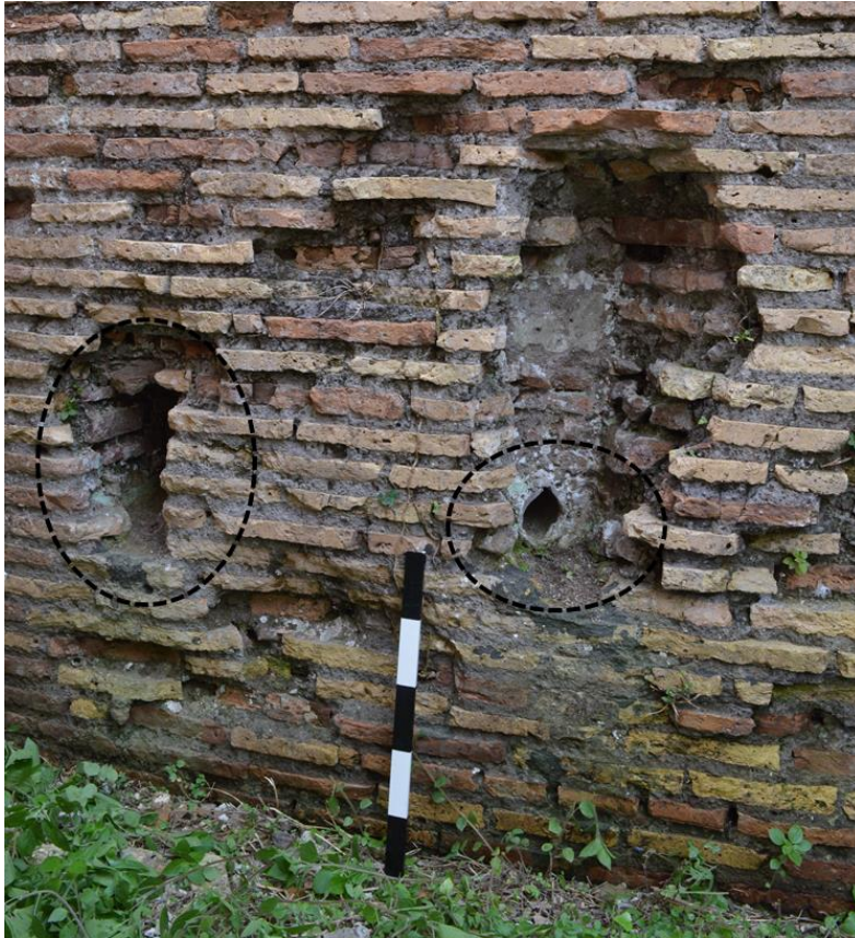
Figure 4.136: Looking south at the north wall of the cistern in building IV, ii, 5. The lead fistula (feature 46) is visible at right, and the channel (feature 107) at left.
