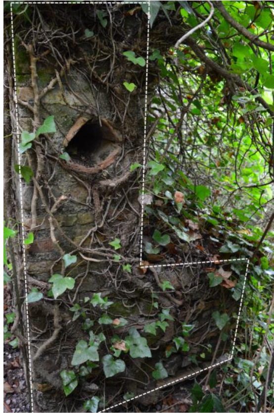
Figure 4.152: West face of the feature 54, showing its L shape, and possible supply line made of two imbrices .
