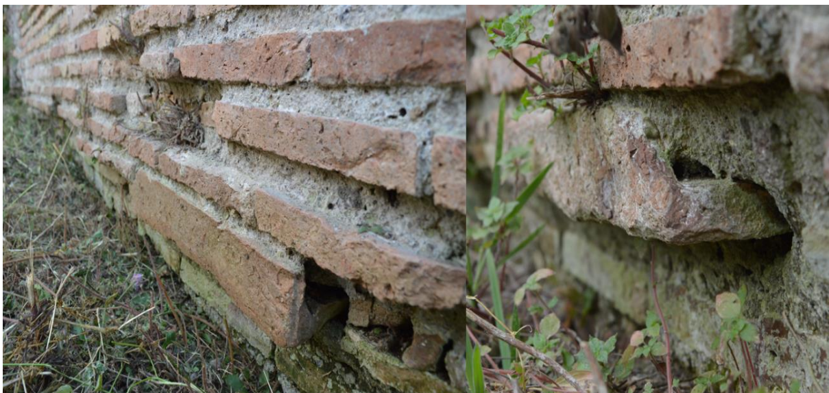
Figure 4.126: View looking east at feature 112, from the northern courtyard of insula IV, ii.
