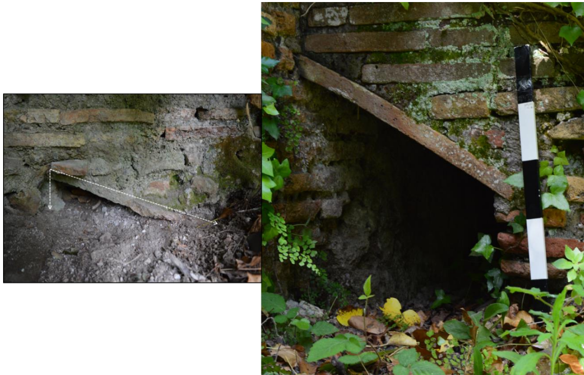
Figure 4.161: Visible features of drain 102 in the northwest corner of room 1 at left. At right, a similar half-cappuccina in the Terme del Faro (IV, ii, 1).
