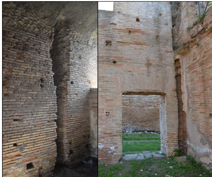
Figure 1.9: Examples of downshafts extending above the ground floor, at left in the Forum baths (I, xii, 6), at right in the Caseggiato dell Serapide (III, x, 3). In the image at right, note the preserved circular ceramic pipe within the masonry shaft.
