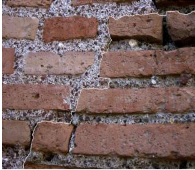
Figure 1.13: A section of mimetically restored wall, with modern repair on the left and ancient masonry on the right (Rinaldi 2012, 24, Fig. 3).
