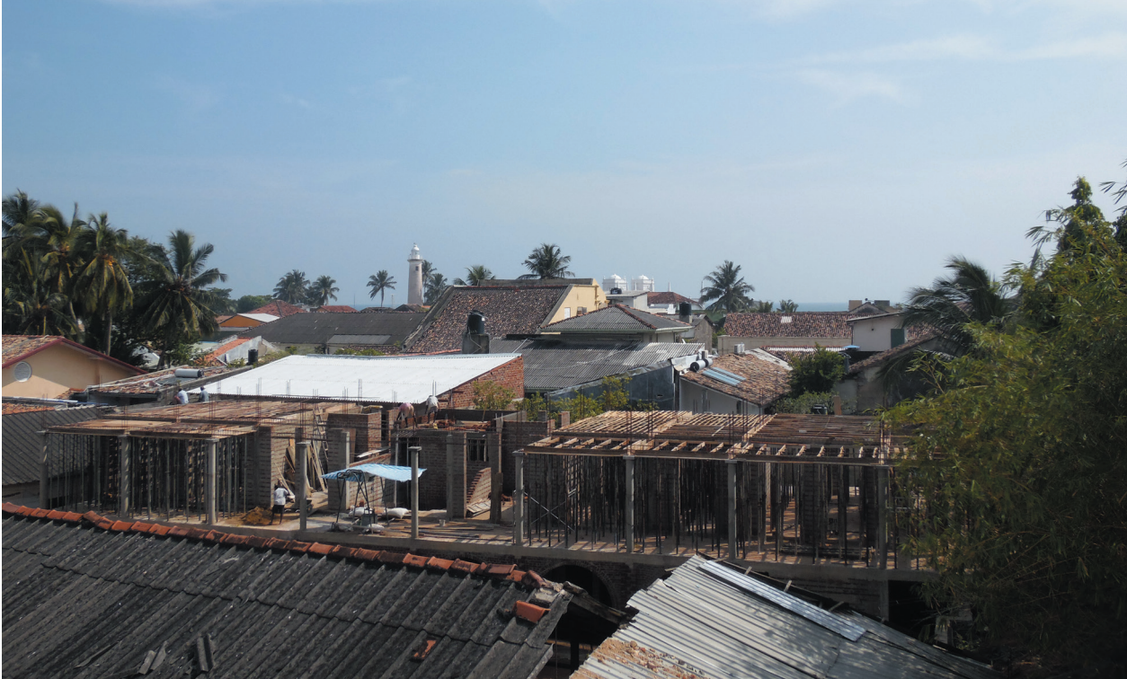
Fig. 271 Permitted building with a third floor, during the construction of its second floor in 2016.
