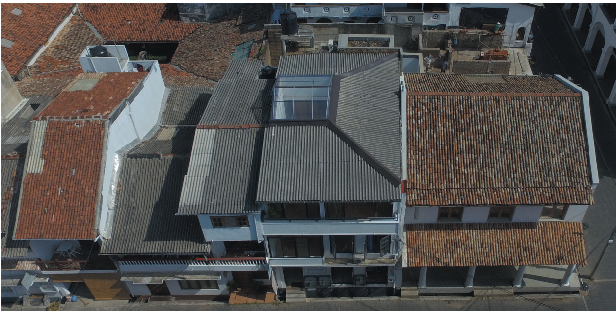
Fig. 134 Difference in the usage of roof materials between approved and "illegal" developments: while half-round tiles over asbestos are used in approved developments (extreme left and right), the rest, in the middle, are covered with the prohibited asbestos.
