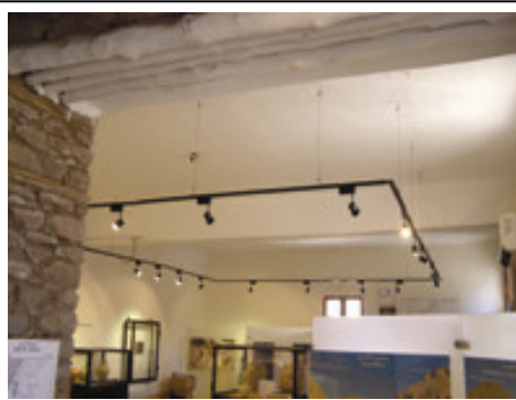
Figure 4.3 Side of a lighting system at the Aqaba Museum. Photo by R. AlGhzawi
