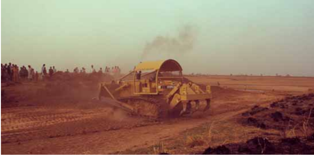
Breaching of the embankment in 1994.
