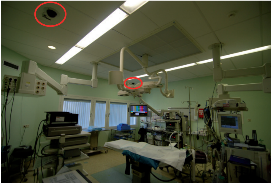
Figure 6.1 Conventional cart-based OR (dome cameras are circled).
