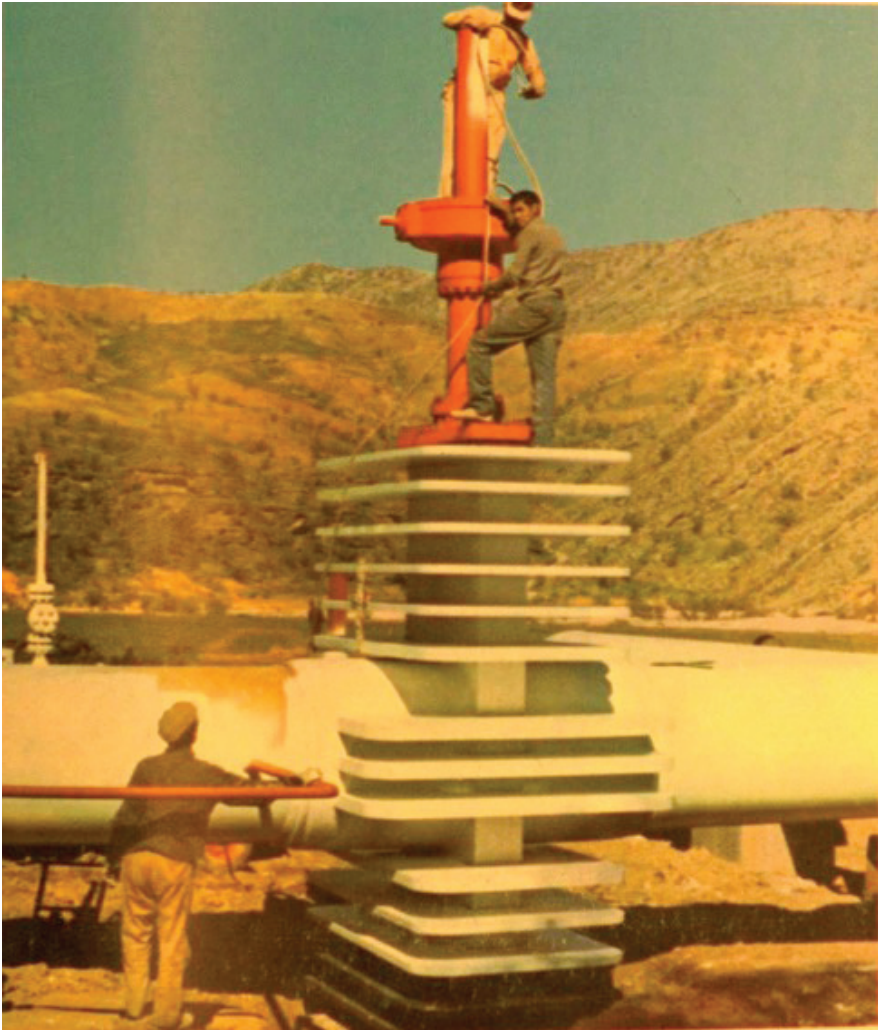
Workers at one of the valves on the main route of the Iranian Gas Trunkline. Published in "NIOC in 1969," National Iranian Oil Company. (NIOC HD 9576. I64 S532a in Library of Congress.)
