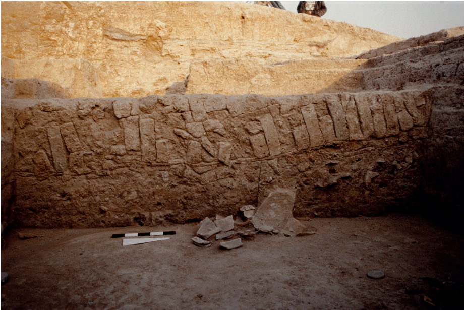
Fig. 3.37: Section of collapsed wall Z in room B of area 2 of the north-eastern sector. Visible on the photograph is that 50 centimetre of soil and refuse had accumulated on the floor before the collapse occurred (photo by P.M.M.G. Akkermans).
