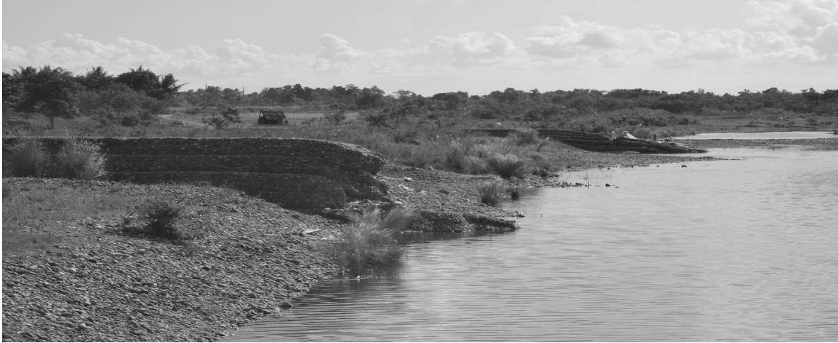
Figure 2: Broken spur dikes and badly repaired dike in San Mateo (Photo by E van Berchum 2012)
