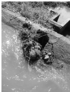
Figure 6: Broken canal lining
