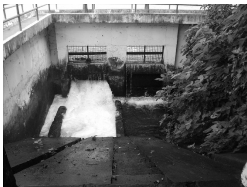
Figure 18: Intake, one gate open
