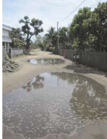
Holes in road, stagnant water
