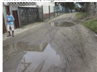
Holes in road, stagnant water
