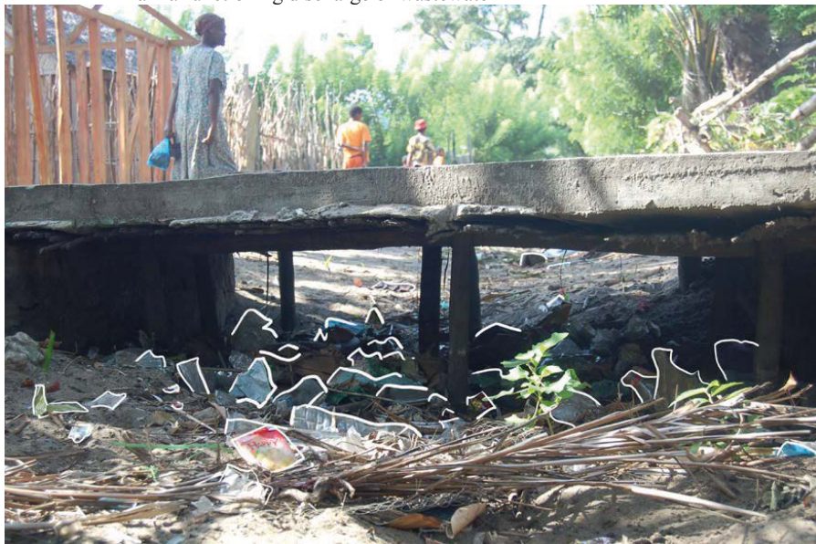
Photo 5.7 People throw waste in the drainage channels and do not maintain them. This results in a malfunctioning discharge of wastewater
