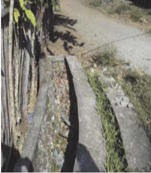
Dirty/ filled gutter along RN
