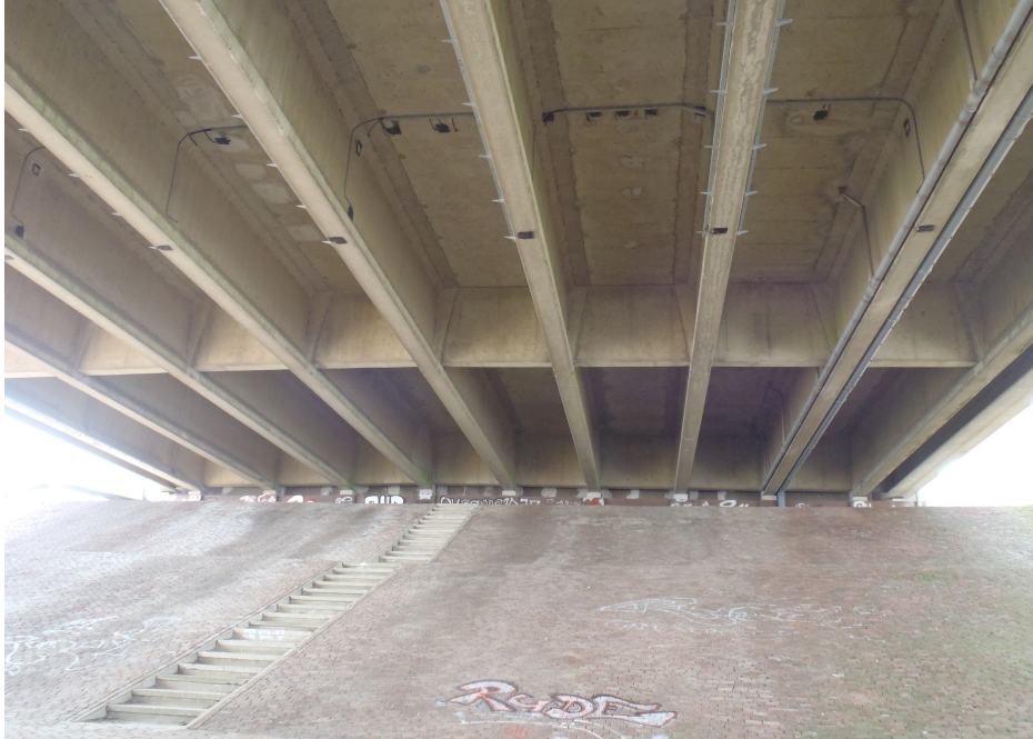
Figure 3.3: Sensor locations of one of the three cross-sections - Sensors are either attached or embedded to the deck and girders of the bridge.
