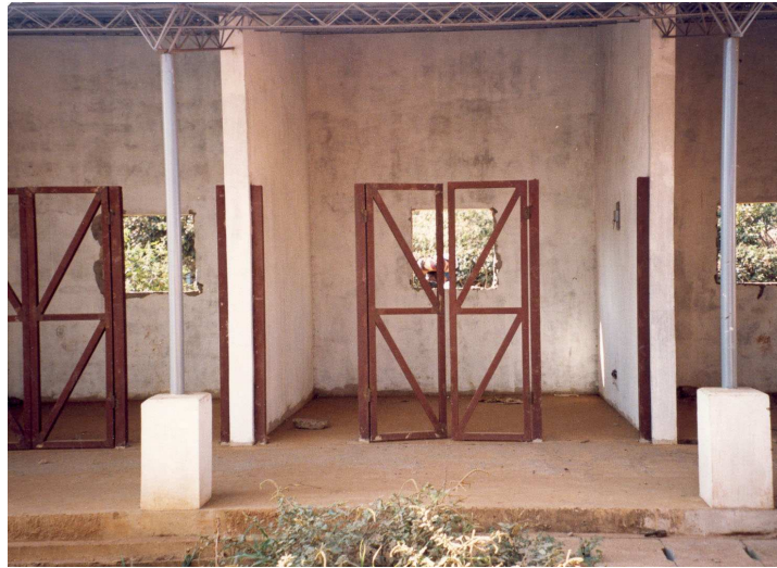
Photo 16 Unfinished market structures at Chilenje
