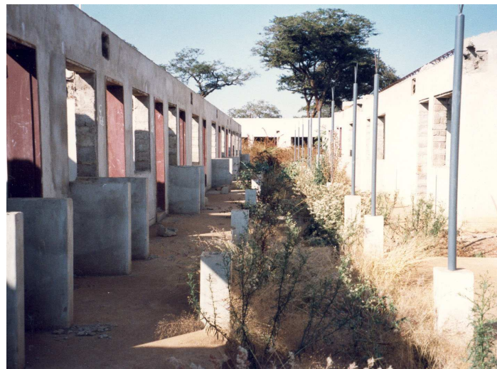
Photo 17 Unfinished market structures at Chilenje
