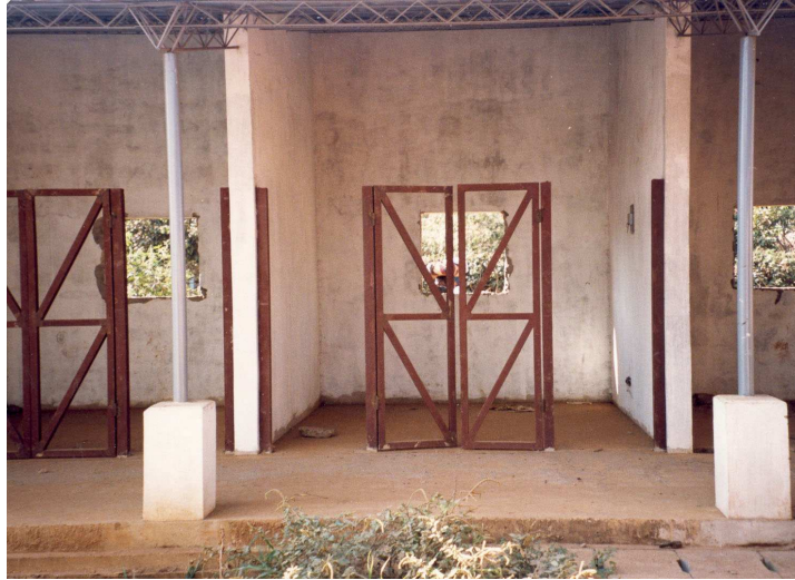
Photo 16 Unfinished market structures at Chilenje
