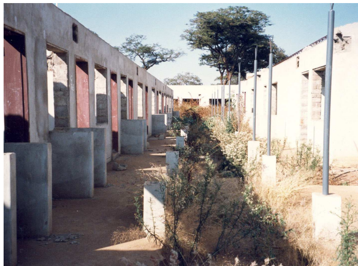
Photo 17 Unfinished market structures at Chilenje
