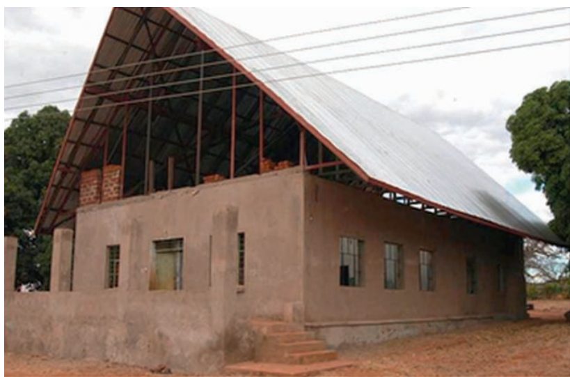
Fig. 9.1 The old Sharma Brothers' Store in Mukuni. When this photograph was taken, it was being renovated by a NGO into a computer centre for the Mukuni community (Source: The Livingstone Museum Archives, Photograph by Fidelity Phiri, June 2010)
