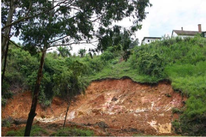
Photo 3.1 & 3.2 Landslide at Up-station at the governor’s residence, August 2009
