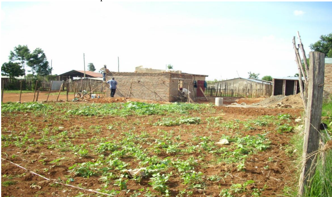
Photo 4.3 A farmer in Langas constructs a rental house on his plot. He previously grew sukuma wiki on the entire plot
