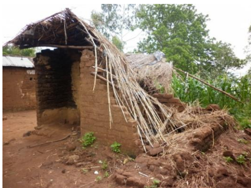
Photo 1: A house in an urban neighborhood of Blantyre, destroyed by the floods.
