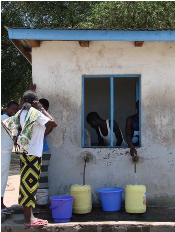
One of the water kiosks operated by the Company [Photo: Dick Foeken, 2008]
