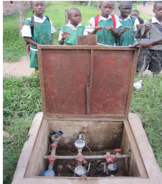
A meter chamber with six connections [Photo: Dick Foeken, 2012]
