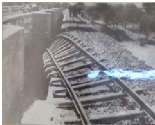
Damaged railroad leading to Agordat, between Hagaz and Dae'rotay.
