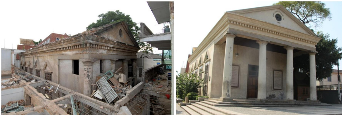
The Union Church before and after repairs. Photos by Chen Yongpeng and author respectively.
