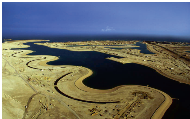
Fig. 17. Photo of Pearl City water channels under development. Photo: La Ala Al Kuwait Real Estate Co. K.S.C., Kuwait.
