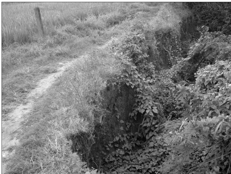
Figure 4: Soil erosion along river bank in Upi
