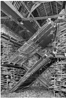
p. 46 Destroyed House Leiden 4 , Leiden (NL), 2016, 226×155 cm, inkjet print on dibond/framed
