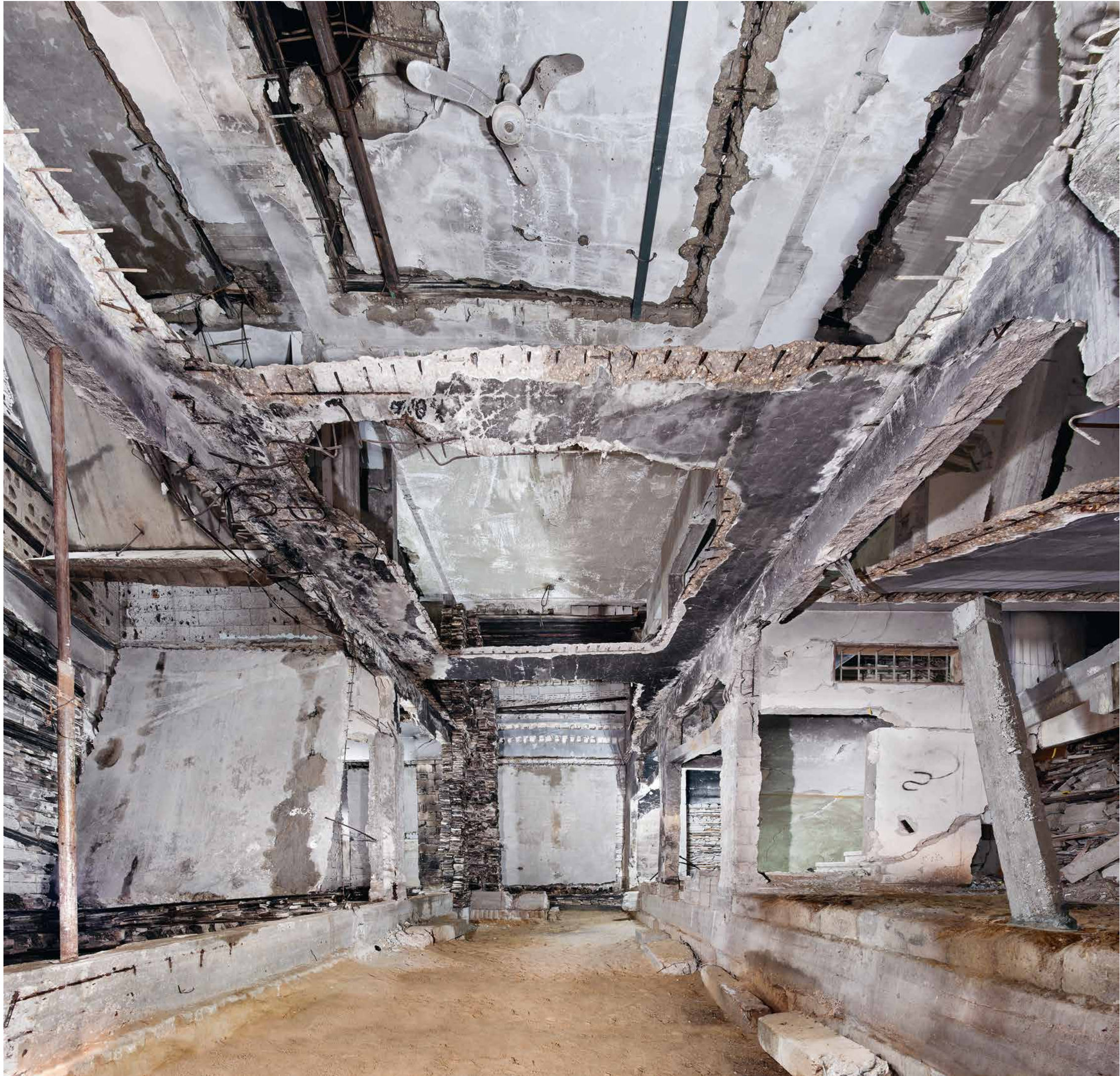
Destroyed House Gaza 5
