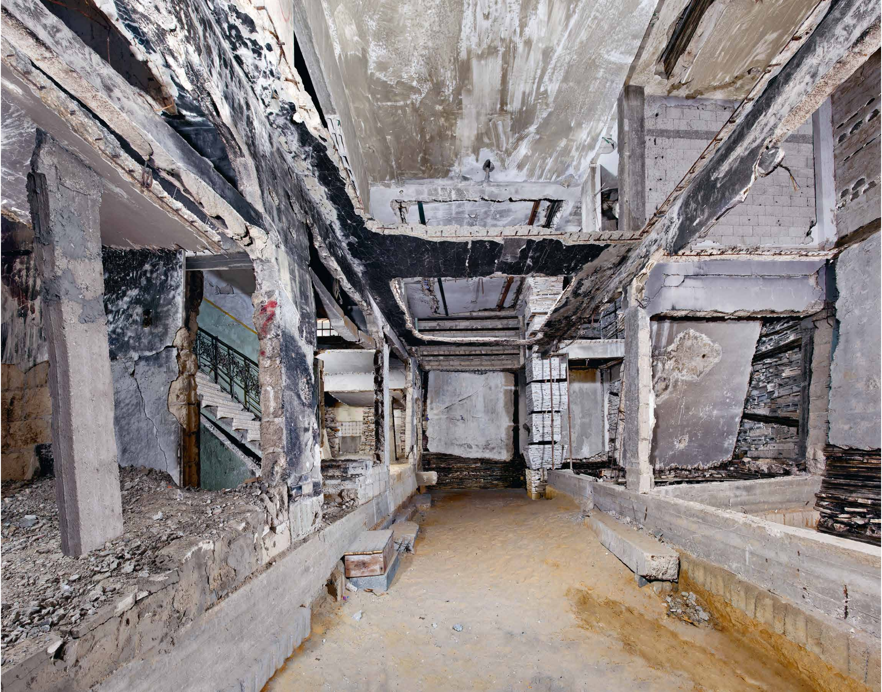
Destroyed House Gaza 4
