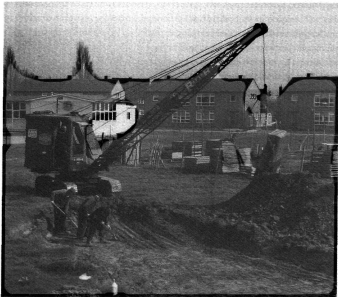
fig. 1.2 Excavations carried out in 1959 by the State Service for Archaeological Investigations in the Netherlands (ROB) at a Neolithic settlement site near Elsloo. This was only a few years after the first attempts had been made to use digging machines in archaeological research. They made it possible to conduct fieldwork on a larger scale.
