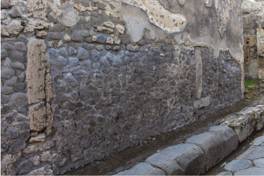
FIGURE 7.3 Pompeii, VII 4, 31. Wall in opus incertum of grey lava with door posts in Sarno stone
